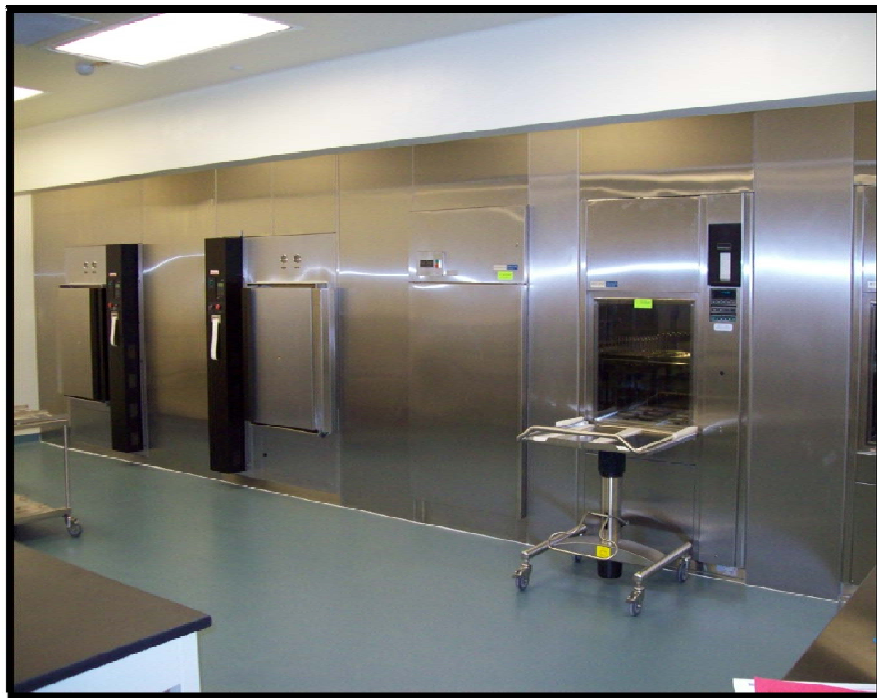
Sterilizers and Dryers with Stainless Steel Mod Wall and Epoxy Finishes
