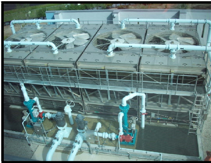
Cooling Towers in Mech. Yard
